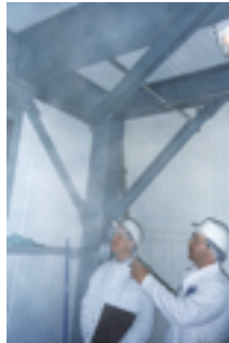
Platform in Food Plant
